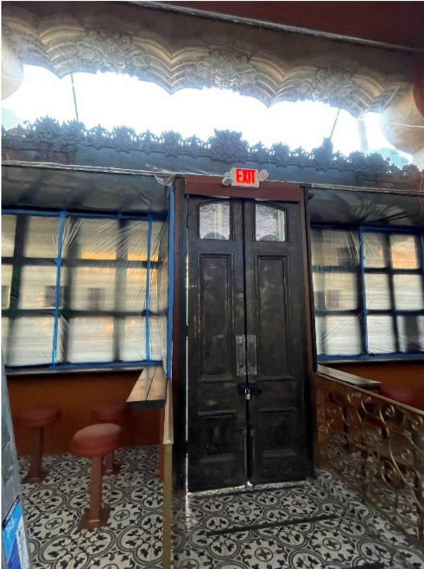
Figure 10 - MFR Report Figure 15 “(Original Doors and Storefront Windows Extant). The patios were enclosed with contemporary storefront, and the original paired wood doors were pushed to the sidewalk to create a flat plane on the primary façade for security reasons in 2004. The interior arches were installed where the original primary façade plane was previously located. SOURCE: Sapphos Environmental, Inc., 2022. NOTE: Metal windows were added in 2001 for security.”
